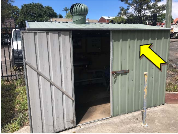
Photo Exterior, throughout, walls and ceiling - 1. suspected lead-containing green upper paint system.
